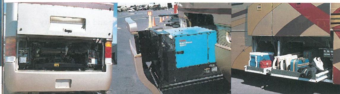
The large rear engine access door with pantograph hinges and struts raises and lowers for easier access to the engine compartment.
