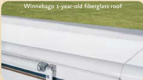
Winnebago 1-year-old fiberglass roof
