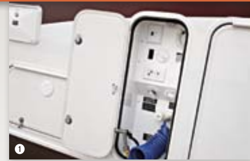
❶ CONTROL CENTER
