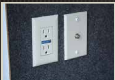
110v outlet and cable outlet conveniently located in the pass-thru storage area.
