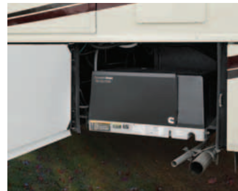
Exterior generator compartment, shown with optional Onan generator.
